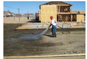
Construction Sites Reduce Construction Dust Comply with Dust Permit Eliminate Dust Fines
